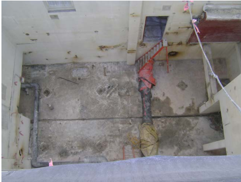
Raw Water Treatment Room Emptied
