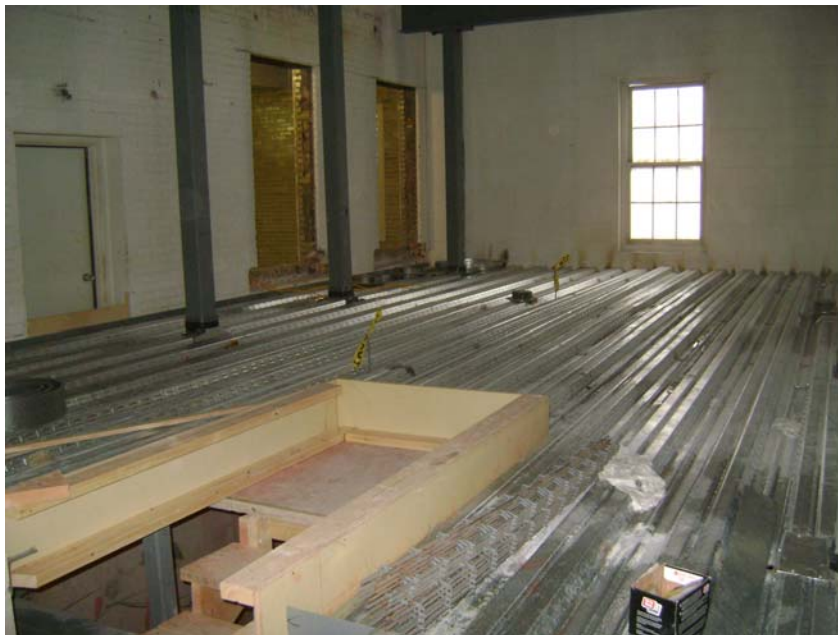
1 st Floor of Raw Water Treatment
